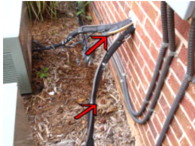
Condensate Discharges too close to house
