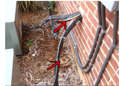
Condensate Discharges too close to house
