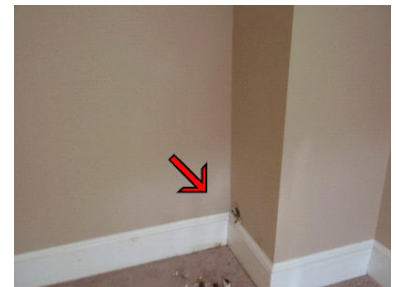
Appears to have water penetration
